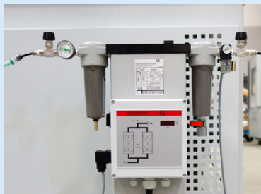
Additional Drying Capacity
